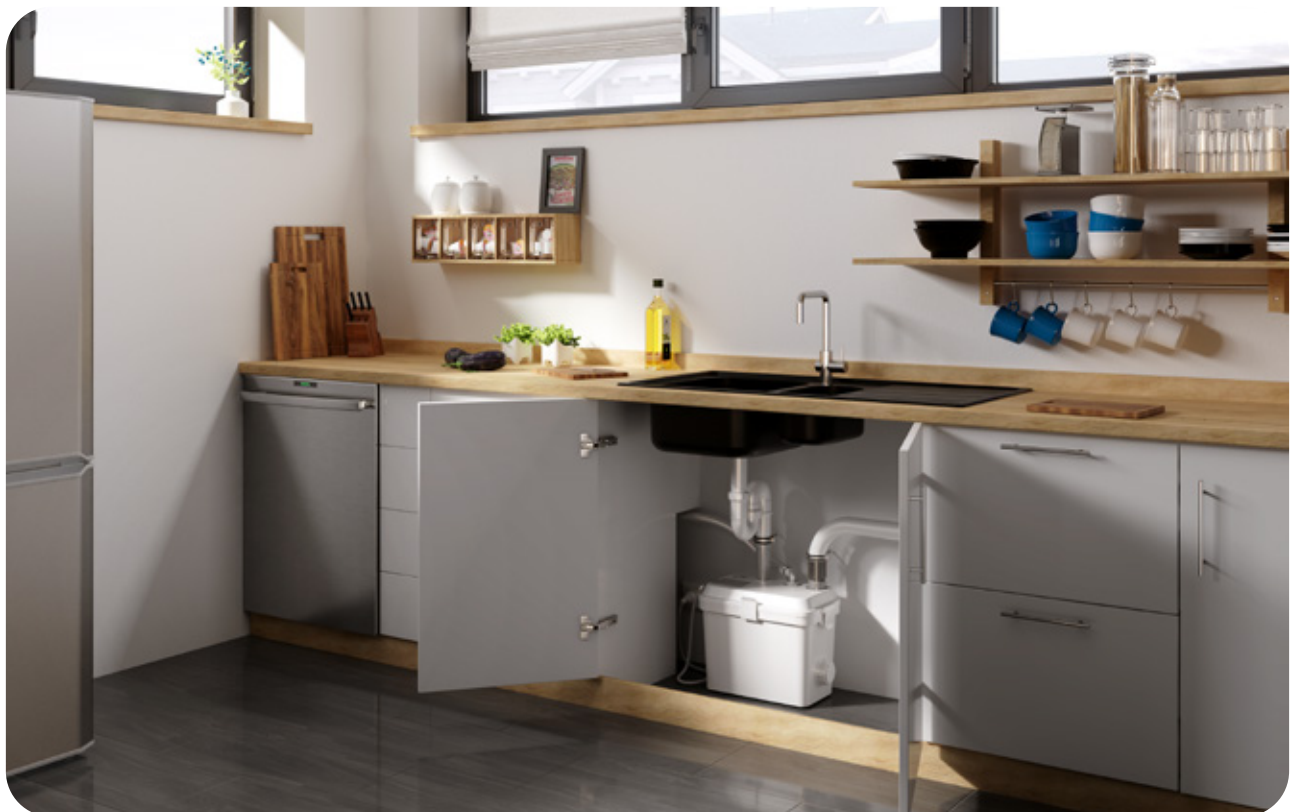
Fig.: SWH 100 in kitchen in basement apartment
